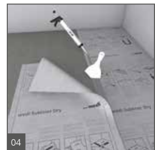
04 The sheets must overlap 50 mm at joints/transitions. Leave these overlapping areas free of any tile adhesive and use tape to keep them folded upward and/or clean. Apply wedi 620 Sealant as a full bed onto the lower mat's seam connection area and press the top overlap flat into the wedi 620 Sealant.
