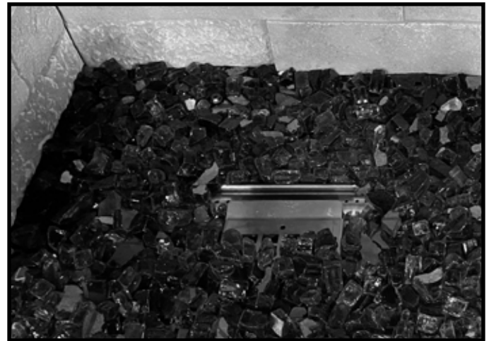
Figure 11.5 Media Placement Jig Removed
