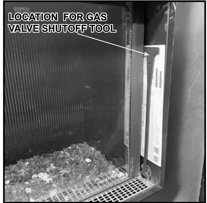
Figure 11.22 Storage Location for Gas Valve Shutoff Tool
