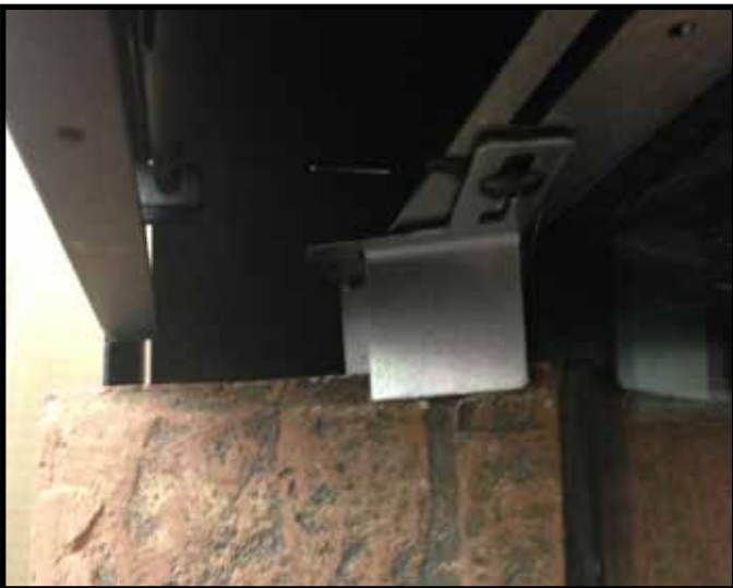
Figure 11.27 Side Refractory Brackets
