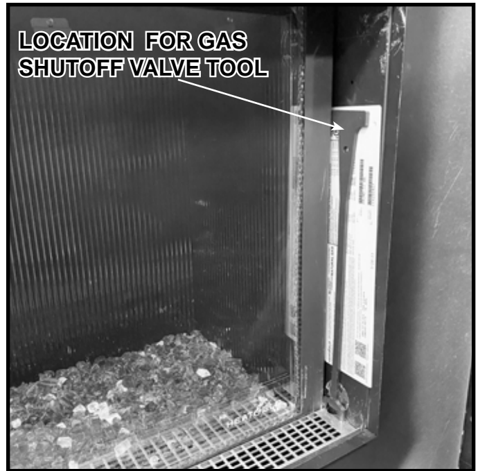
Figure 4.12 Storage Location for Gas Shutoff Valve Tool
