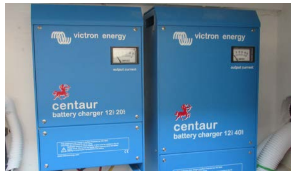
Battery chargers (typical)
