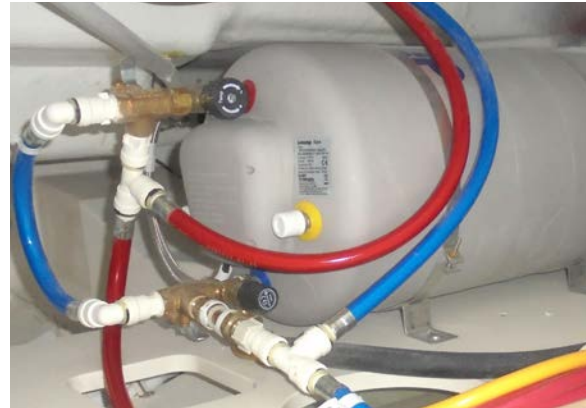
Water heater (typical)
