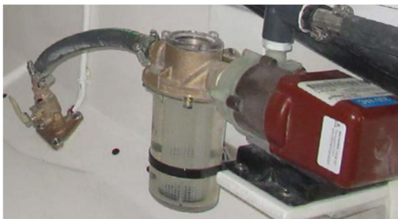
Air conditioning valve, strainer, and pump
