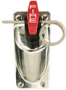
Fire system manual discharge pull
