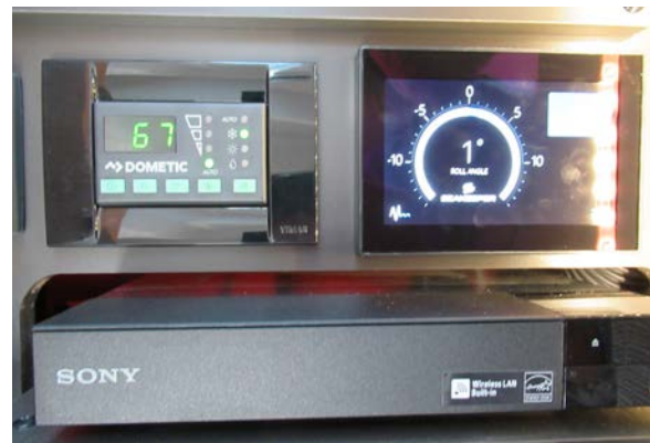
AC distribution panel (typical)
