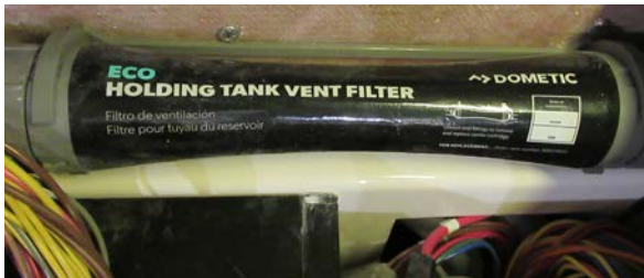
Tank vent filter, in the engine room on top of the holding tank
