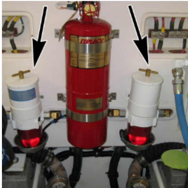
Figure 7-1: Engine room fuel filters/water separators.
