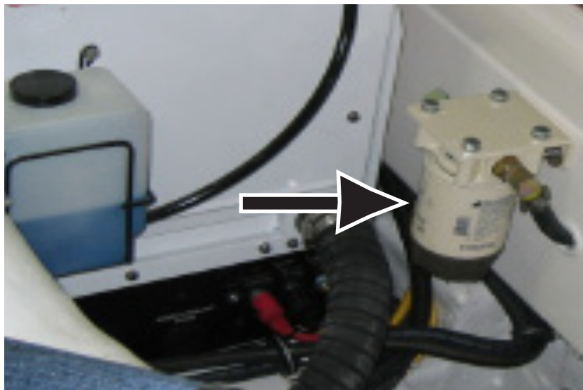
Figure 7-5: Generator fuel filter, located on the port aft engine room bulkhead.
