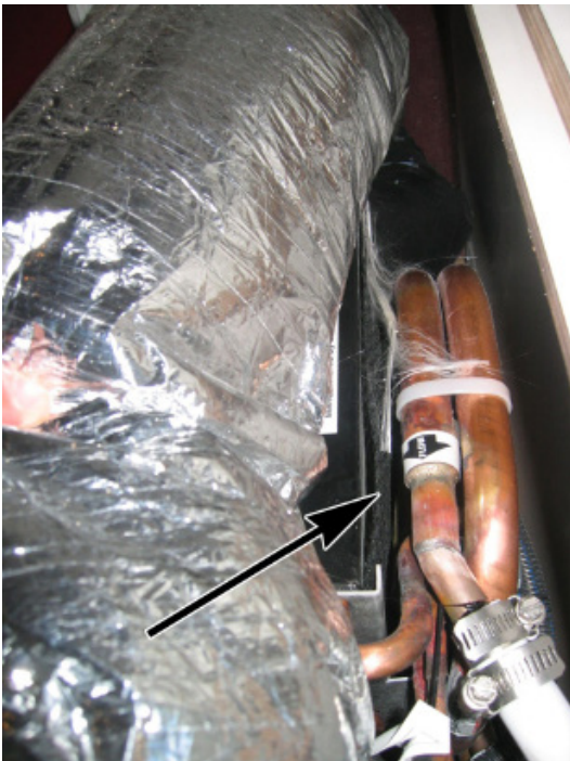
Figure 7-11: The A/C unit below the master stateroom aft berth storage. The arrow points to the mesh filter.
