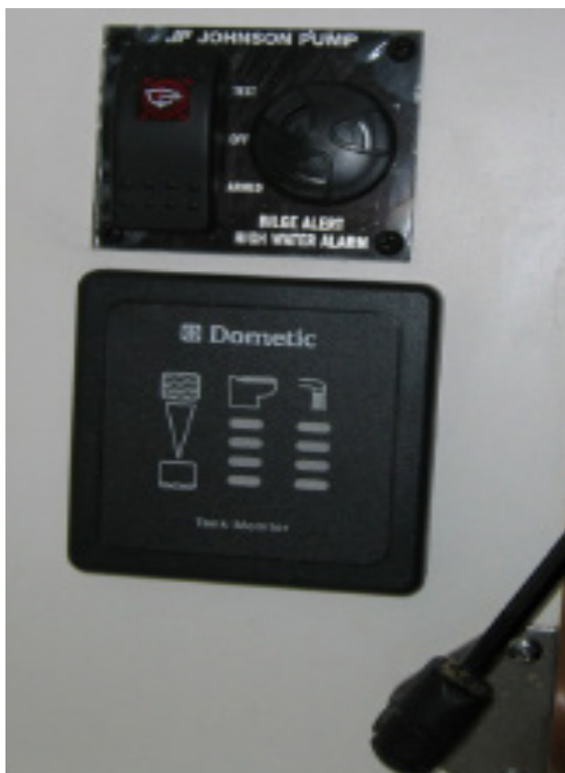
Figure 2-3: Inside of the upper hullside dinette cabinet. Above: the Johnson Pump is a bilge alert that sounds an alarm when water reaches a level above the bilge pumps. Refer to the manufacturers information for operation guidelines. Below: the Dometic® Tank Monitor Panel - refer to section 2.2.2 for details.
