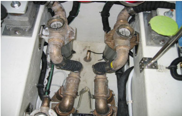
Figure 3-2: Engine raw water seacocks and strainers.
