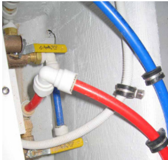
Figure 6-4: Water Heater Valves Open.
