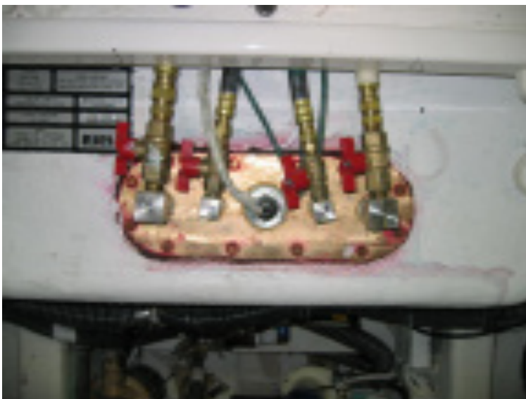
Figure 7-2: Aft fuel tank fuel valves, located below the aft centerline floor hatch.
