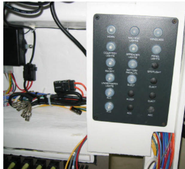
Figure 1-5: The helm breaker panel behind the console.
