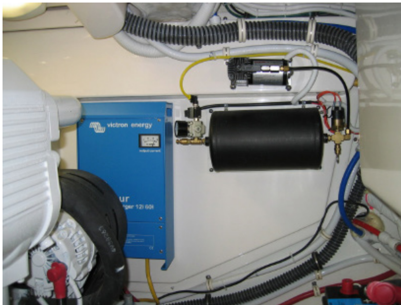
Figure 3-6: Starboard side forward engine room bulkhead. Battery charger (left), Horn compressor (right).
