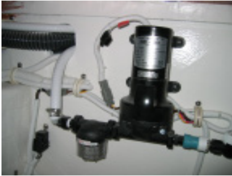
Figure 7-6: Fresh water filter and pump.
