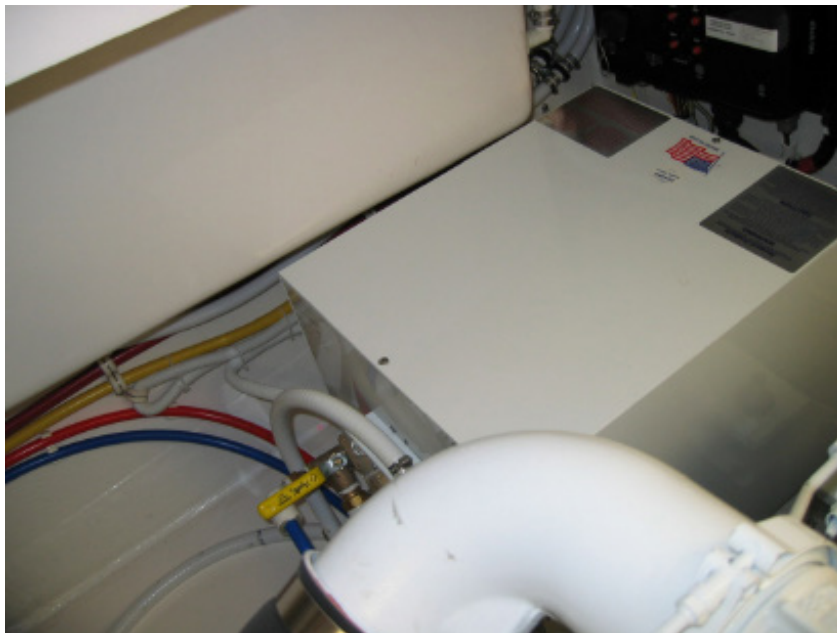
Figure 3-7: Water heater on port.
