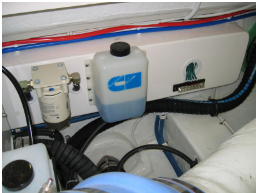
Figure 3-9: Aft of the port engine. Generator fuel filter (left).
