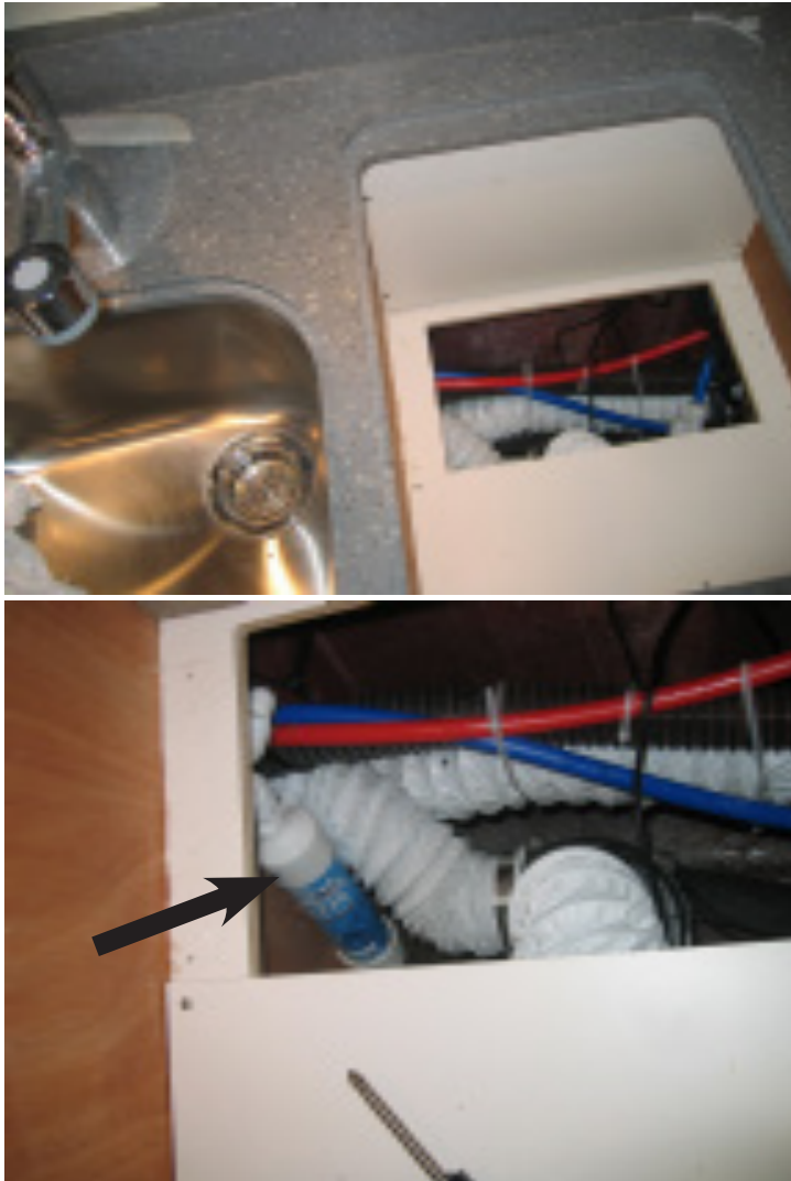
Figure 7-7: Access the galley inline freshwater filter by first removing the Corian® lid forward of the galley sink. Next remove the panel in the outboard storage compartment. The filter is on the aft side of the opening (arrow in lower picture).
