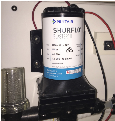
Typical raw water strainer (left) and pump
