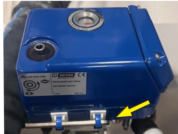
Generator seacock valve with manual override lever
