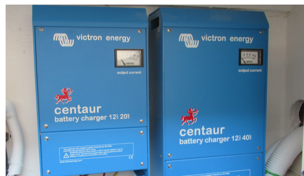
Battery chargers (typical)
