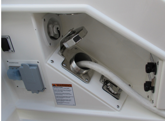
Starboard aft shorepower locker
