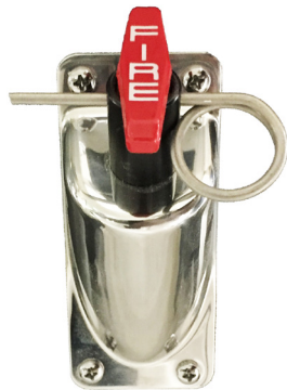
Fire system manual discharge pull
