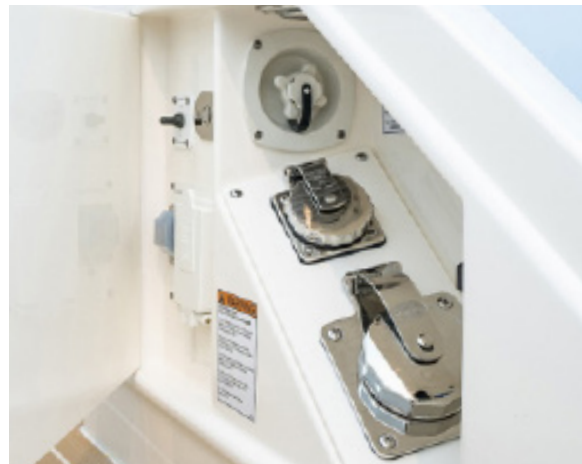
Aft shorepower cabinet
