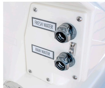
Optional fresh and raw washdown inlets, in the starboard shorepower locker
