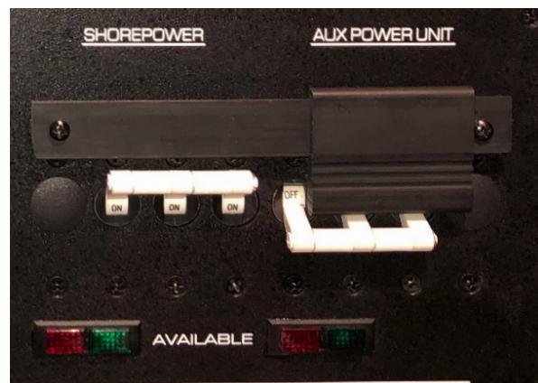
Shore power and aux power (generator) switch and polarity indicator lights
