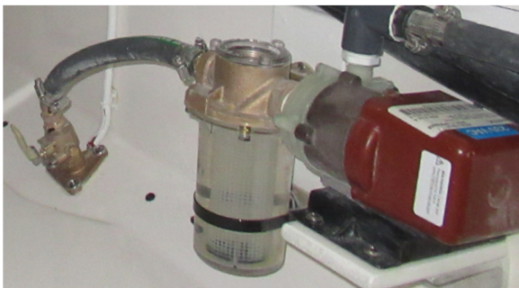
Air conditioning pump, strainer, and valve
