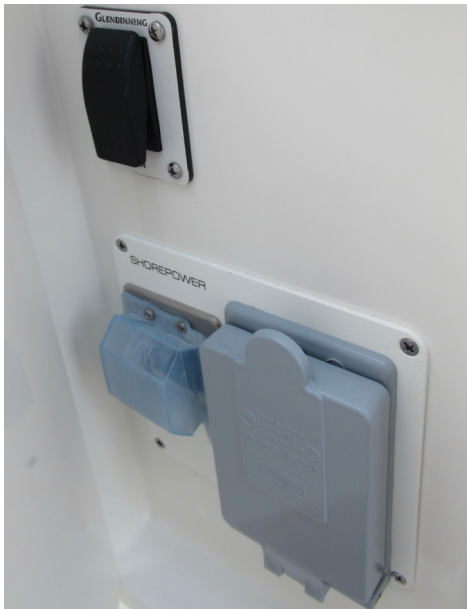
Shore power breaker, ELCI outlet, and shore power cable reel switch (behind cover)
