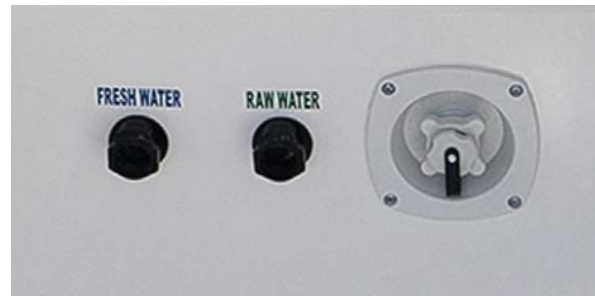
Water connection cabinet
