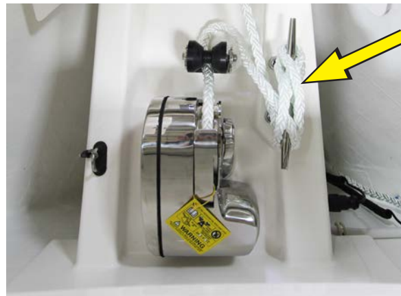
Windlass and anchor rode cleat (typical)
