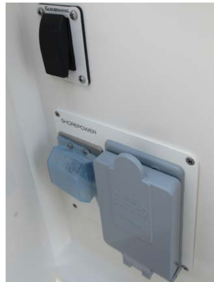
Shore power breaker, ELCI outlet, and shore power cable reel switch (behind cover)
