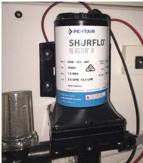
Typical raw water strainer (left) and pump
