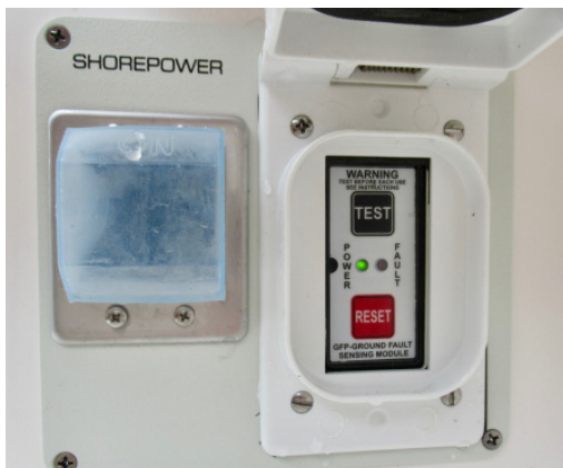
Shore power breaker and ELCI ground fault sensing module
