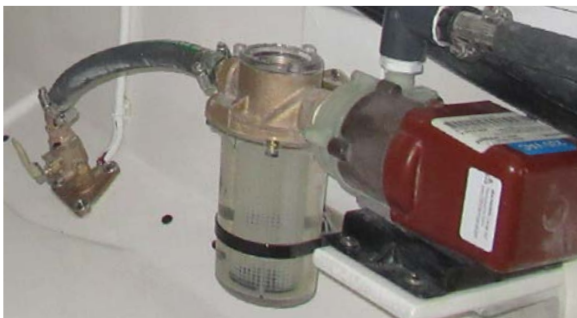
Air conditioning pump, strainer, and valve
