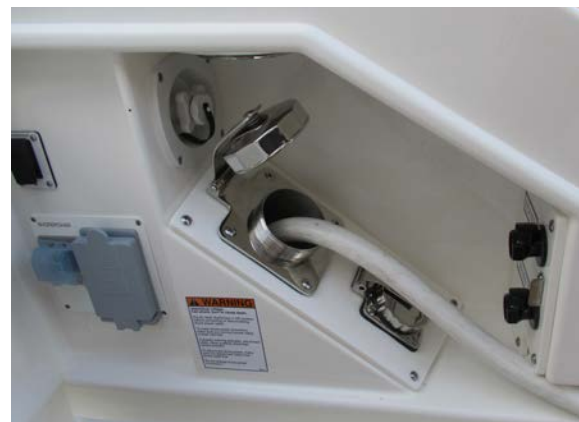
Starboard aft shorepower locker
