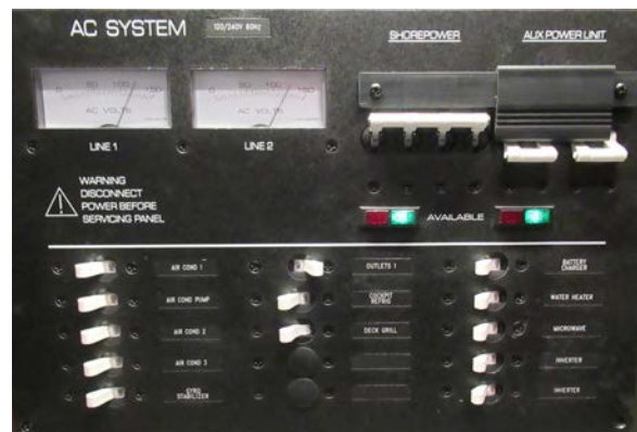
AC distribution panel (typical)
