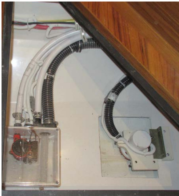
Shower sump box and bilge pump
