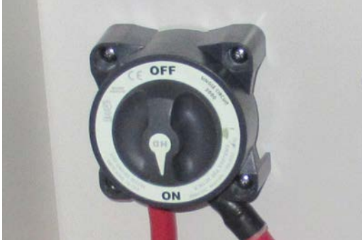
Bow thruster battery switch
