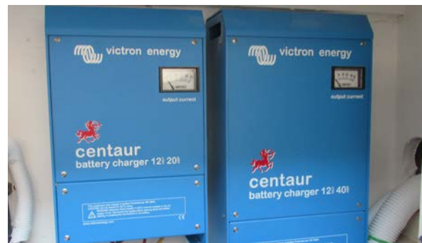
Battery chargers (typical)
