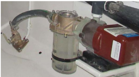
Air conditioning pump, strainer, and valve
