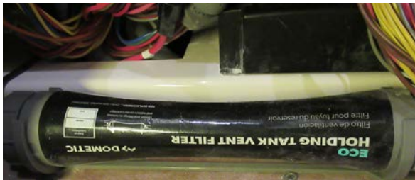
Tank vent filter, in the engine room near the holding tank
