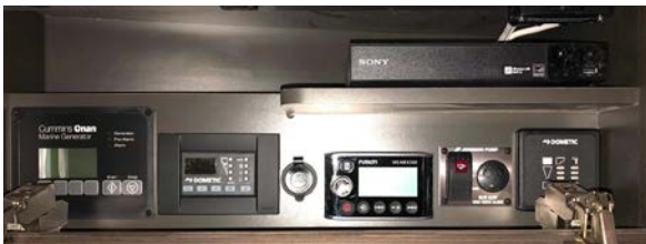
Starboard cabin lower electrical cabinet
