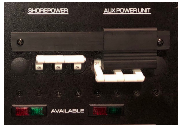
Shore power and aux power/generator select switch and polarity indicator lights (typical)
