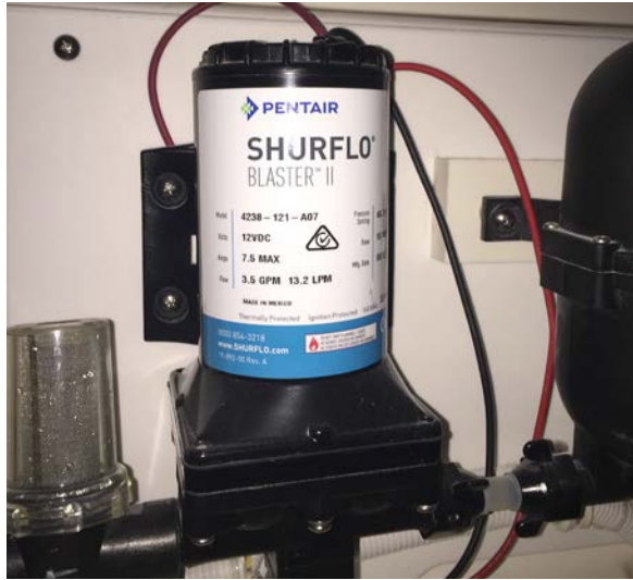
Raw water strainer (left) and pump (typical)
