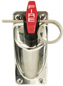
Fire system manual discharge pull
