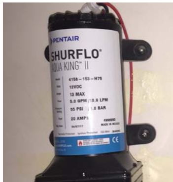
Fresh water pump, in the mechanical space
