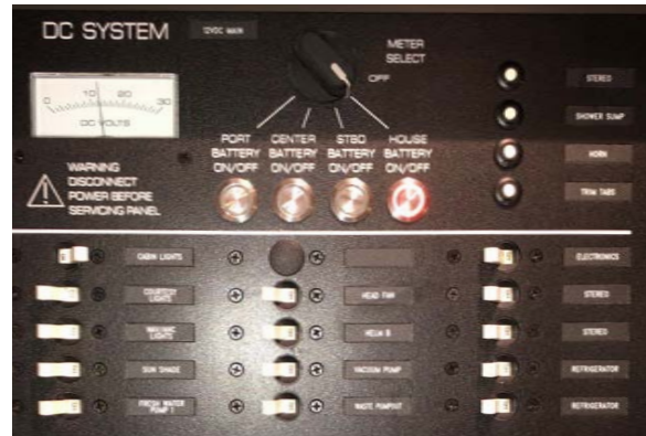
DC distribution panel
