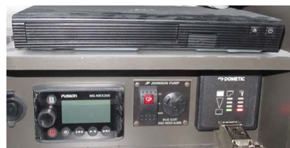
Cabin lower electrical cabinet
