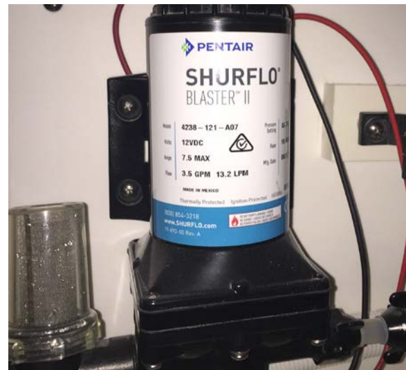
Typical raw water strainer (left) and pump
