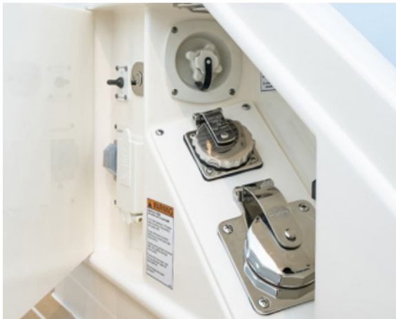
Aft shorepower cabinet
