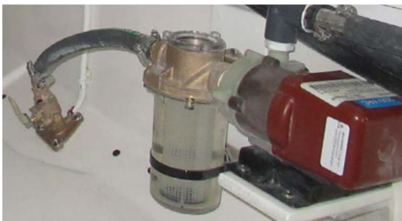
Air conditioning valve, strainer, and pump
