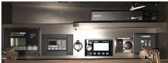
Starboard cabin lower electrical cabinet
