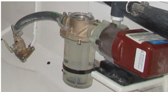
Air conditioning pump, strainer, and valve
