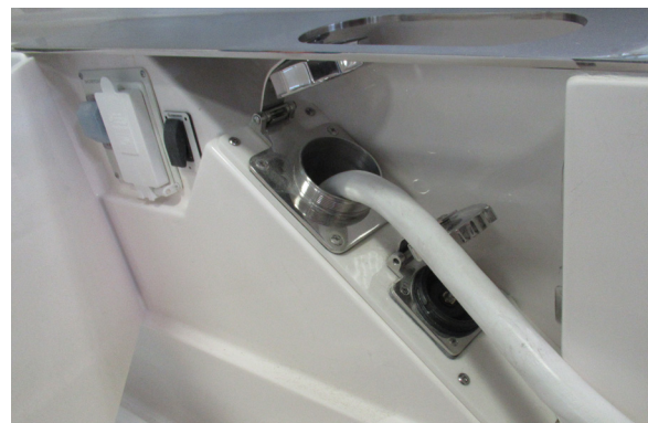
Main shorepower breakers and inlets in aft starboard shorepower locker
