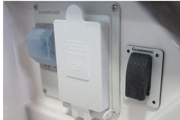
Shore power breaker, GFI outlet, and shore power cable reel switch
