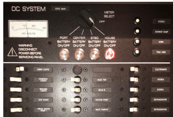
DC distribution panel
