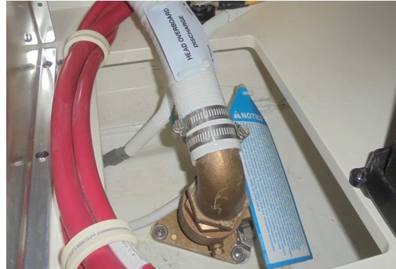
Overboard waste discharge seacock
