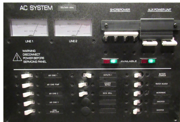
AC distribution panel (typical)
