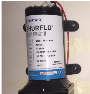
Fresh water pump, in the mechanical space
