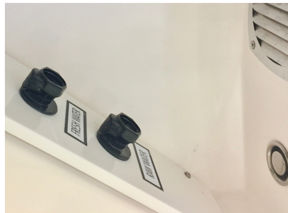
Water connection locker with optional fresh and raw washdown inlets
