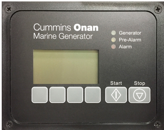
Remote generator control panel, in the port companionway lower cabinet
