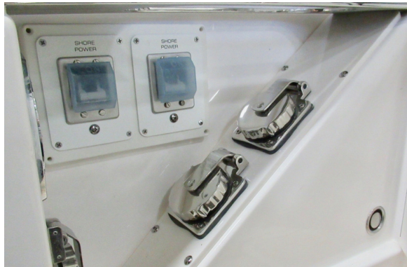
Main shorepower breakers and inlets in aft starboard shorepower locker
