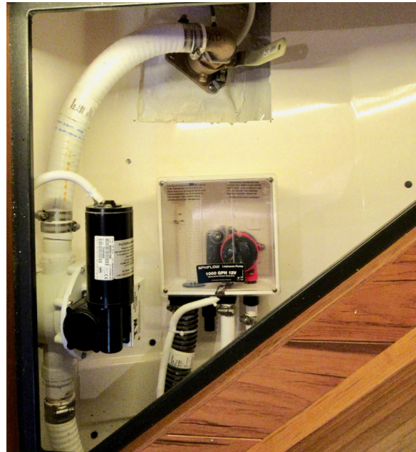
Waste pump (left), overboard discharge valve (top), shower sump box (bottom)
