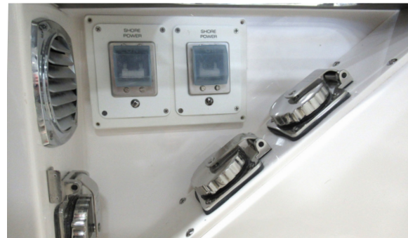
Shore power cabinet
