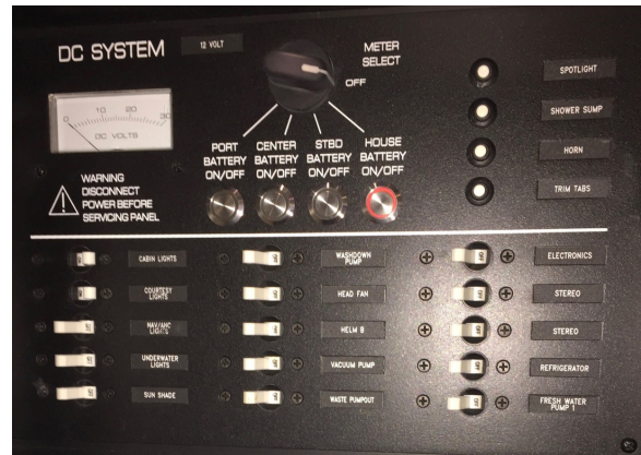
DC distribution panel
