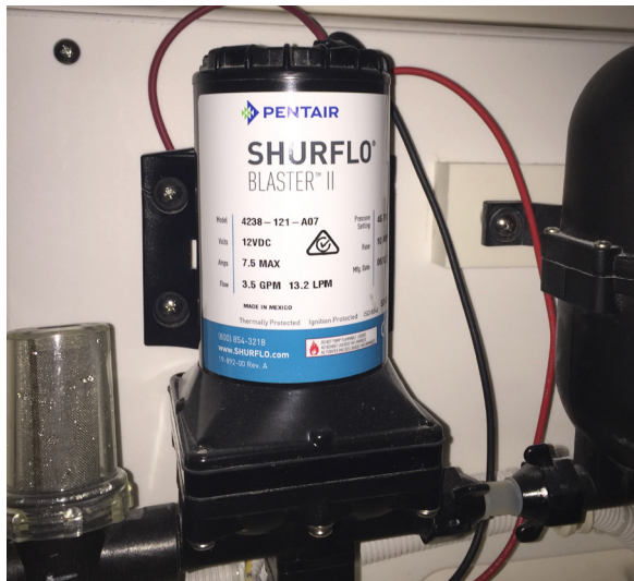
Raw water strainer (left) and pump, in the aft starboard mechanical space
