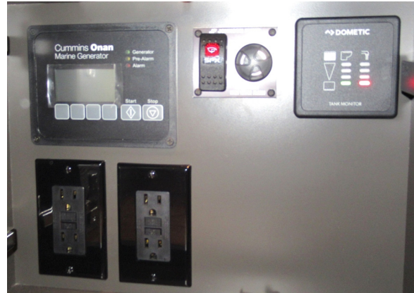
Generator control; high water alarm; holding tank monitor; and outlets, in the port companionway lower cabinet
