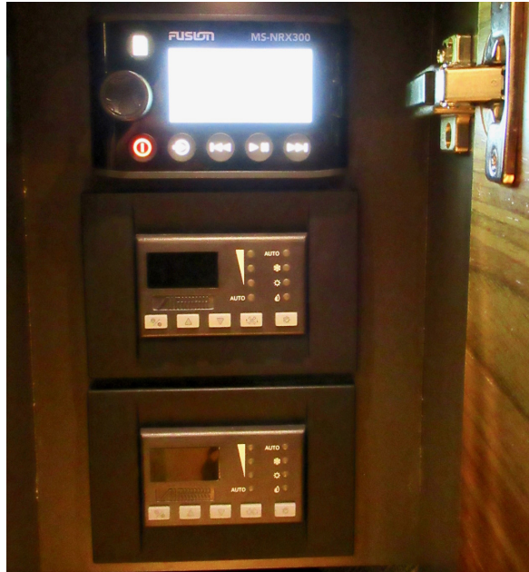
Climate control panels and stereo remote control panel, located in the starboard berth cabinet
