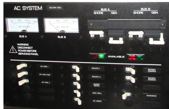
AC distribution panel
