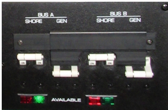
Shore power and generator indicator lights, on the AC distribution panel
