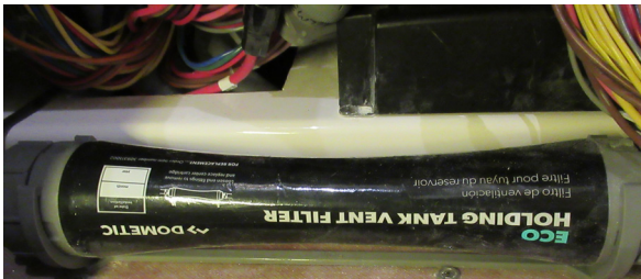
Tank vent air filter, behind access panel in head compartment
