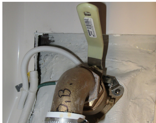
Waste discharge seacock, under cabin floor hatch
