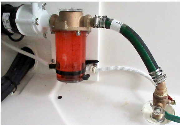
Air conditioning pump, strainer, and valve
