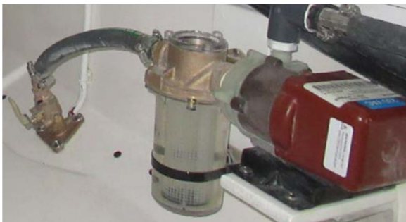
Air conditioning valve, strainer, and pump
