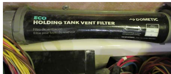
Tank vent filter, in the mechanical space near the holding tank
