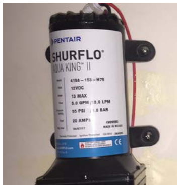
Fresh water pump, in the mechanical space
