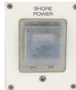
Shore power breaker
