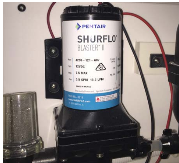
Typical raw water strainer (left) and pump
