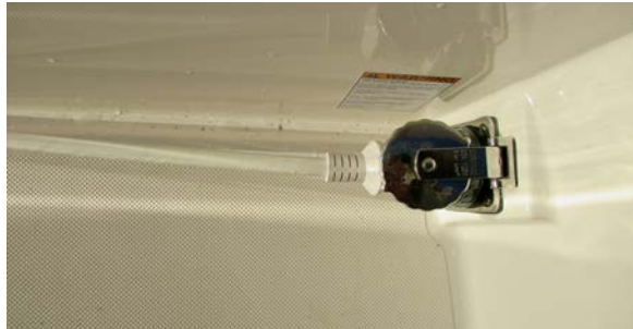
Shore power inlet, outboard of refrigerator
