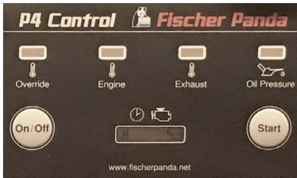
Remote generator control panel
