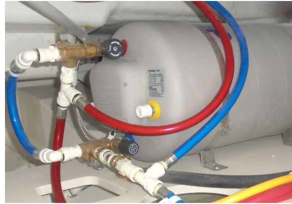
Water heater (typical)
