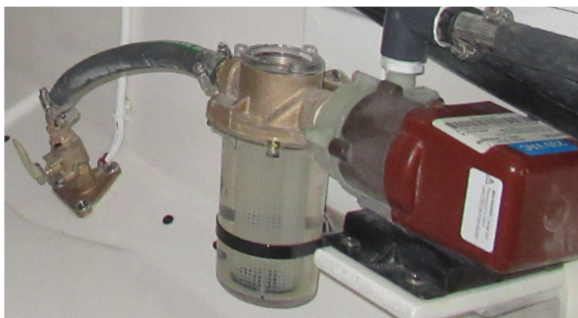
Air conditioning valve, strainer, and pump
