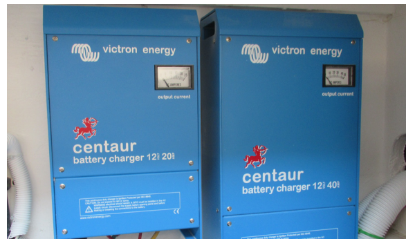
Battery chargers (typical)
