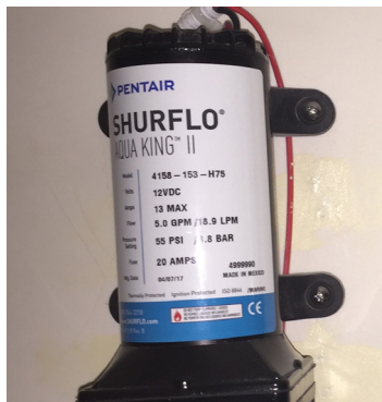
Fresh water pump, in the mechanical space
