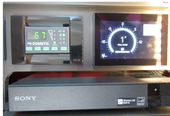
AC distribution panel (typical)
