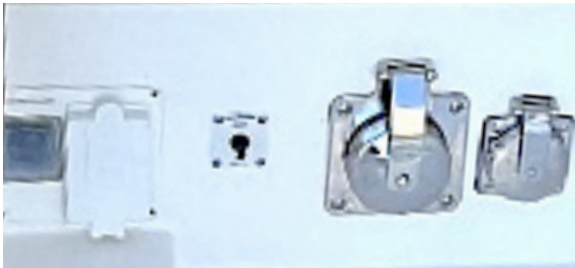
Aft starboard shorepower locker
