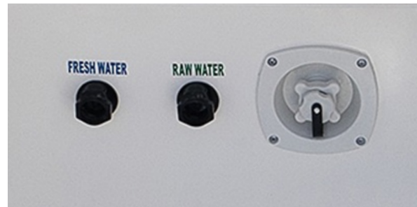
Water connection cabinet
