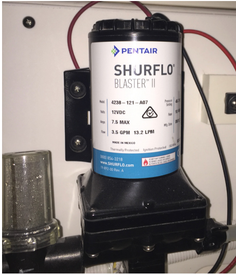
Typical raw water strainer (left) and pump
