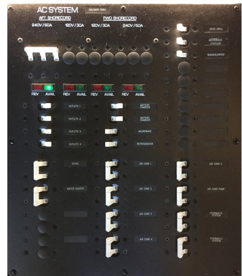
Figure 4-2: AC Distribution Panel
