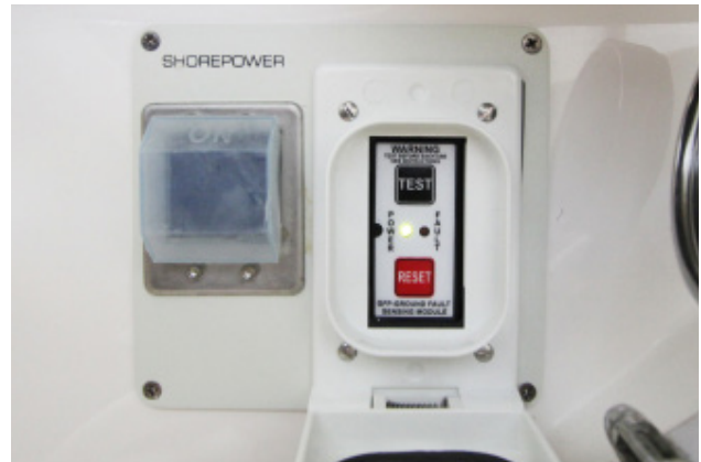
Figure 1-10: Breaker & ELCI reset
