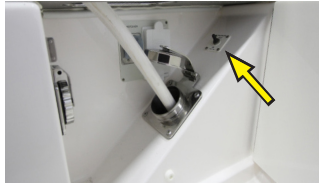
Figure 5-2: Aft port shore power locker and cable master switch
