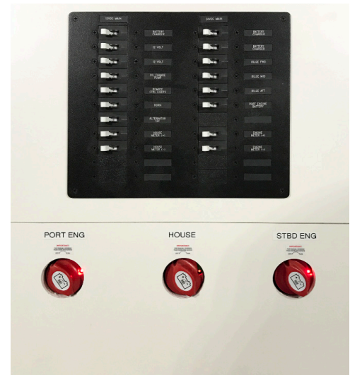
Figure 4-1: Master DC Panel
