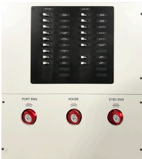
Figure 3-2: Master DC Panel and main battery bank switches
