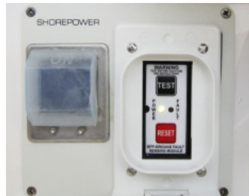
Figure 5-1: Shore power breaker and selector switch
