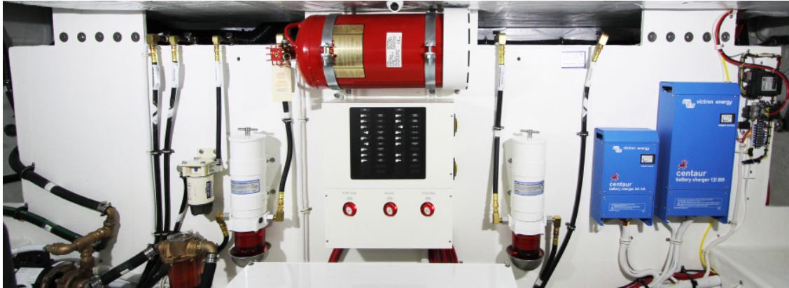
Figure 3-1: Forward engine room bulkhead
