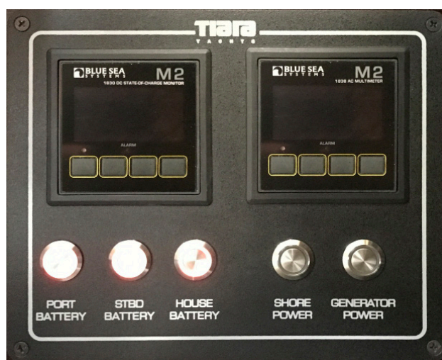
Figure 1-1: Power control panel
