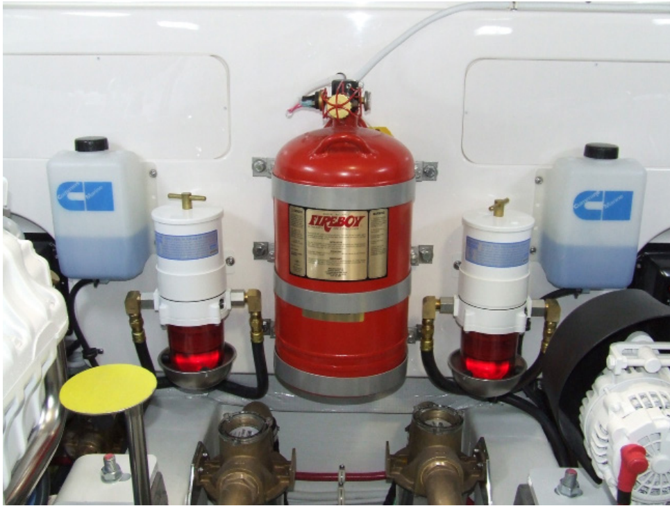
Figure 7-1: Engine room fuel filters/water separators.
