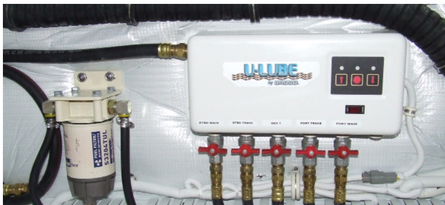
Figure 7-5: Generator fuel filter, located on the starboard aft engine room bulkhead.
