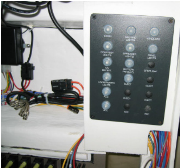
Figure 1-5: The helm breaker panel behind the console.
