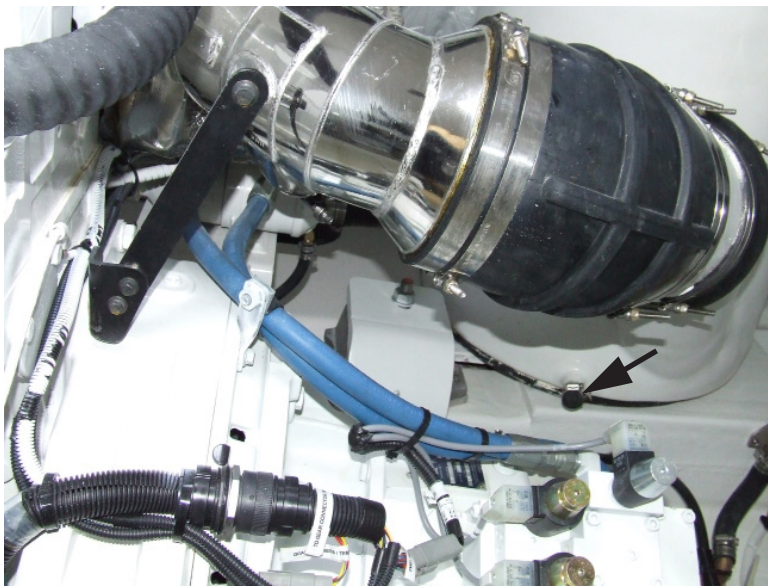
Figure 8-2: Port engine muffler plug shown. The muffler plugs are accessed through the port and starboard floor hatches.
