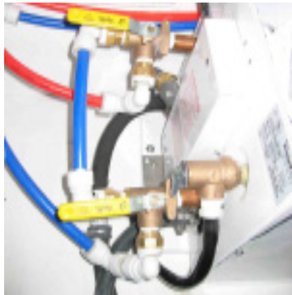
Figure 6-4: Water Heater Valves Open.
