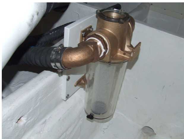
Figure 3-4: Port side raw water strainer shown in the aft bilge area. Zeus pod drive location only.
