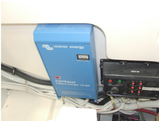
Figure 3-7: Port side forward engine room bulkhead. Battery charger (left), and port engine Cummins Vessel Interface Panel (right). In Zeus applications the Battery Charger is forward on starboard.
