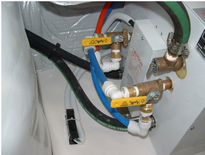
Figure 3-9: Water heater on port.
