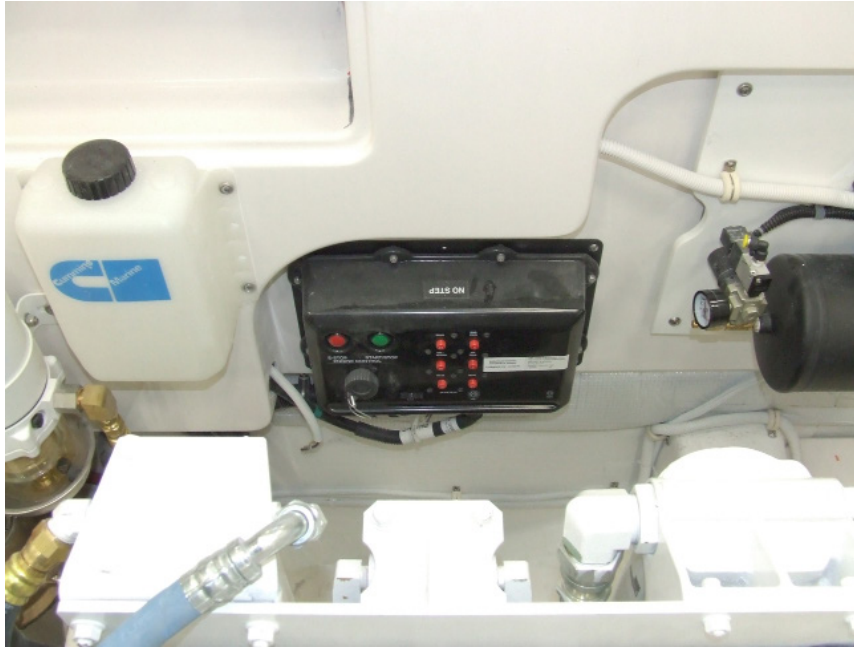
Figure 3-8: Starboard engine coolant overflow (left), horn compressor (right), Cummins panel (center).
