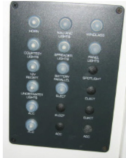
Figure 4-2: Helm Breaker Panel. behind the console.
