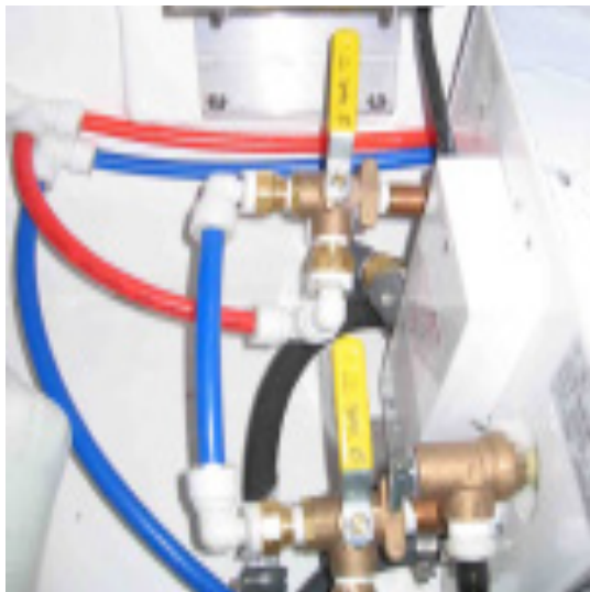
Figure 6-3: Water Heater Valves Closed.
