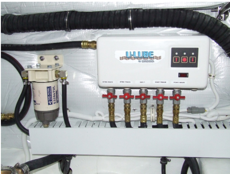
Figure 3-5: Aft of the starboard engine. Generator fuel water separator and oil changer. The oil changer is aft of the port engine in Zues applications.
