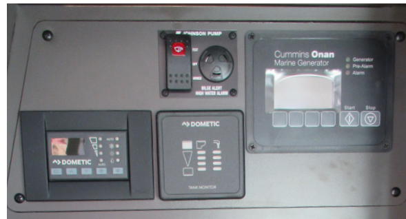
Water alarm; generator control panel; climate control panel; and waste/water tank level indicators
