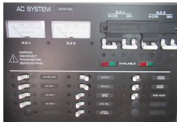
AC distribution panel
