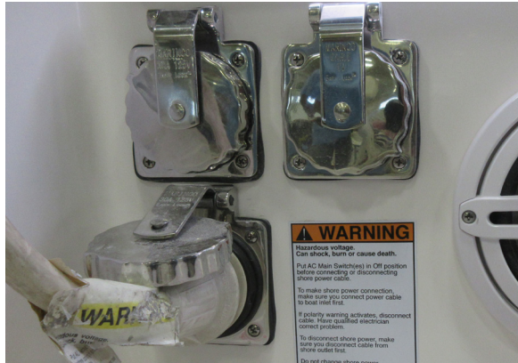
Shore power and cable TV inlets
