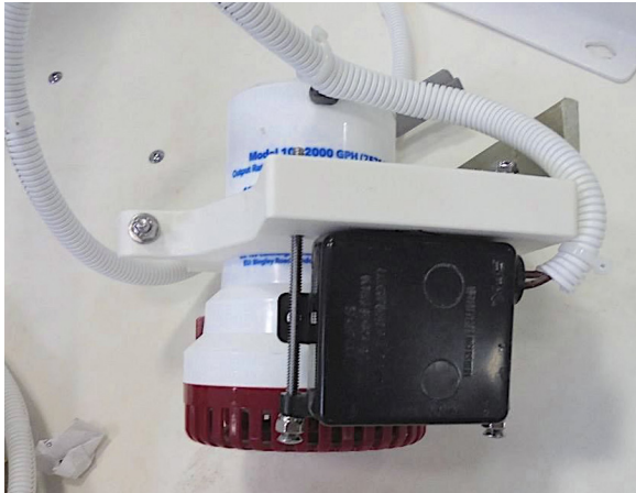
Typical bilge pump and float switch (right)
