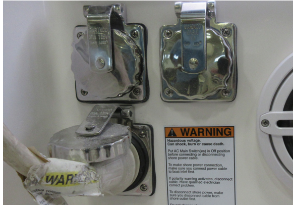
Shore power and cable TV inlets
