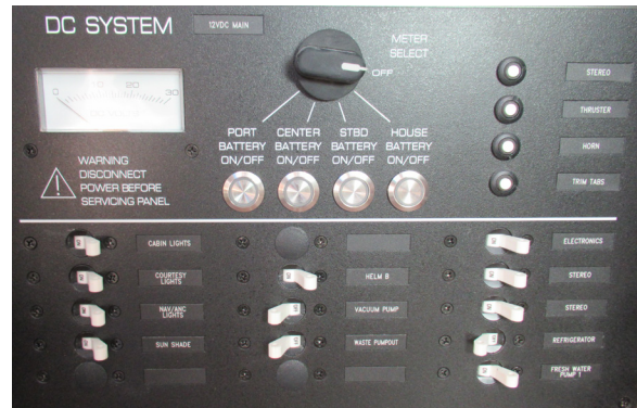
DC distribution panel
