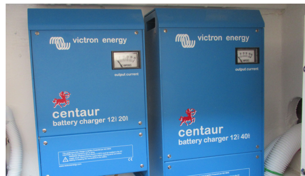
Battery chargers (typical)
