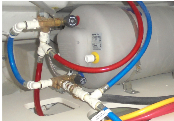
Water heater (typical)
