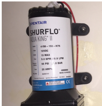
Fresh water pump, in the mechanical space
