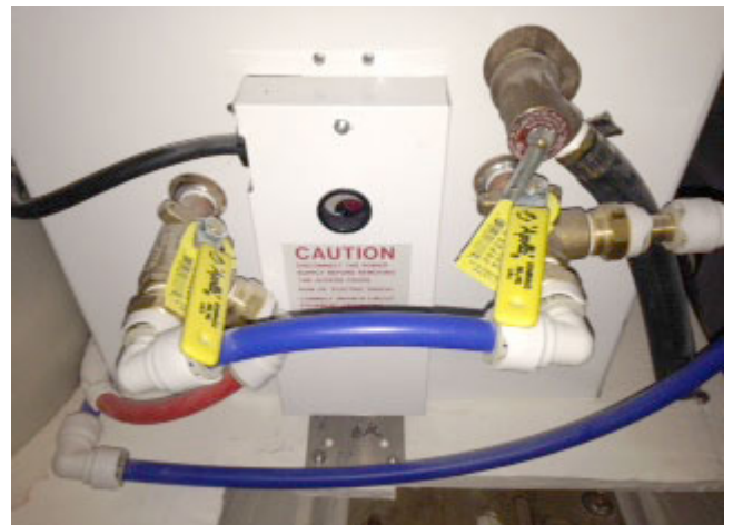
Figure 6-3: Water Heater Valves Open.
