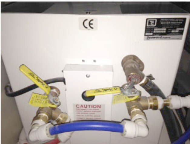
Figure 6-2: Water Heater Valves Closed.
