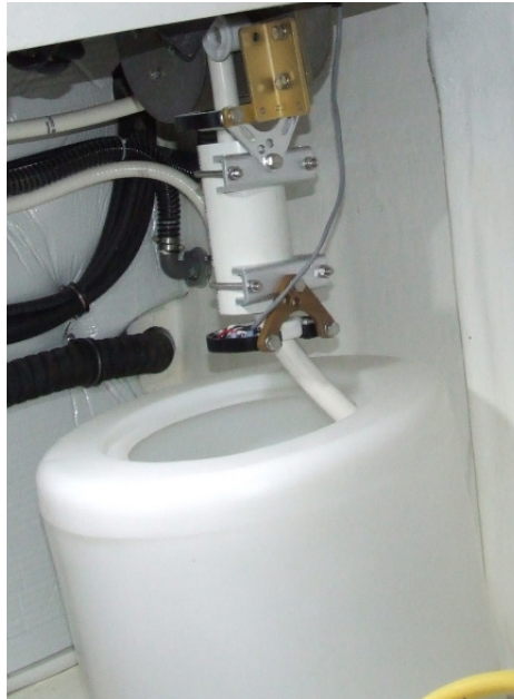
Figure 3-2: Storage bucket for the aft 50A, 240V shore power cable, outboard on port.
