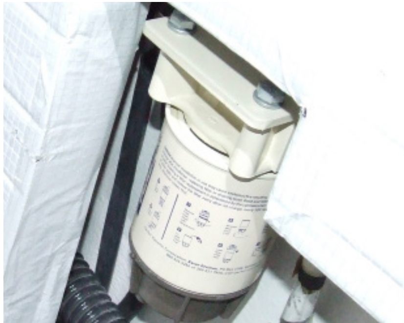
Figure 7-1: Generator fuel filter, located on the forward port engine room bulkhead.
