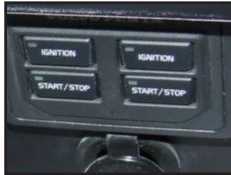
Figure 5-4: Volvo ignition controls below the outboard flip up cover, just aft of the controls at the helm.
