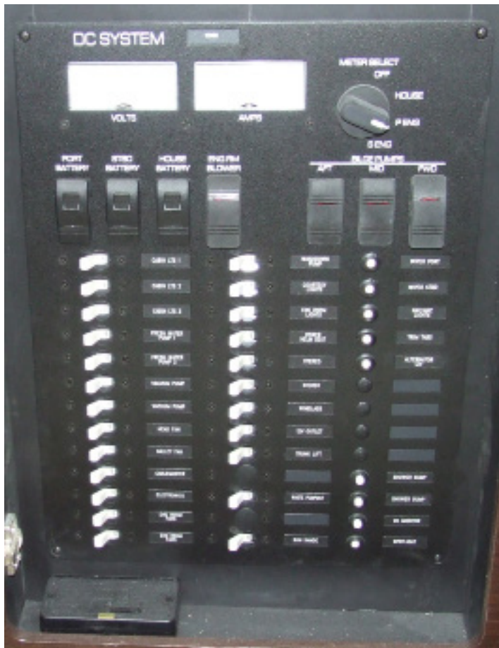
Figure 4-1: D.C. System Panel.
