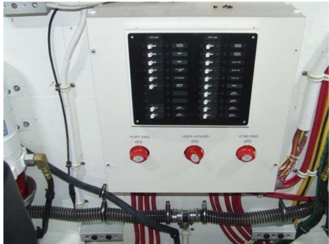
Figure 3-1: Centerline, forward engine room - The Electrical Panel Box & Battery Bank Switches.
