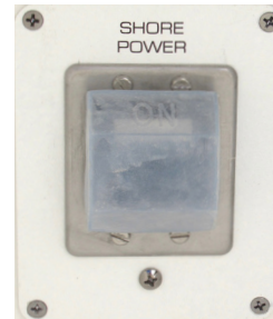
Shore power breaker
