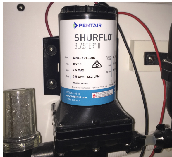
Typical raw water strainer (left) and pump
