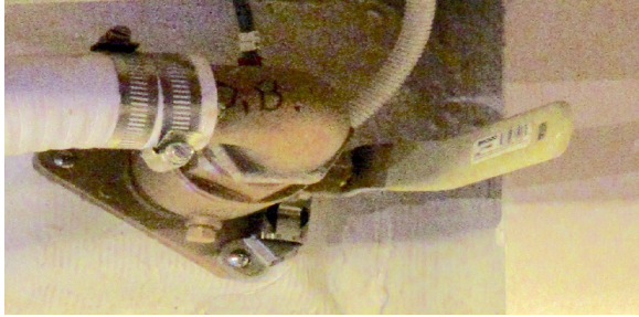
The waste discharge seacock, located at the end of the discharge hose.
