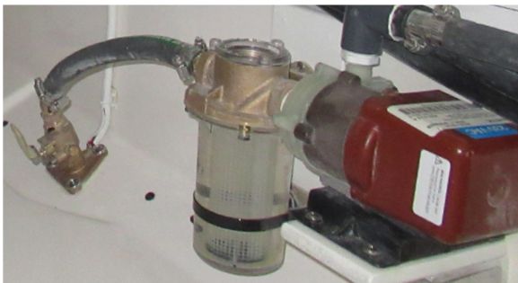
Air conditioning valve, strainer, and pump
