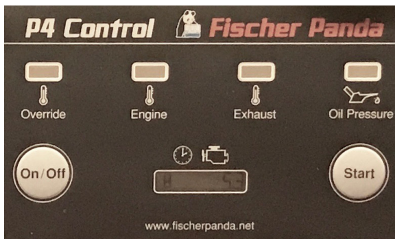
Remote generator control panel
