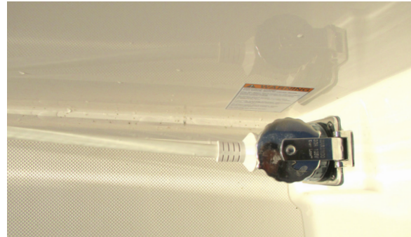
Shore power inlet
