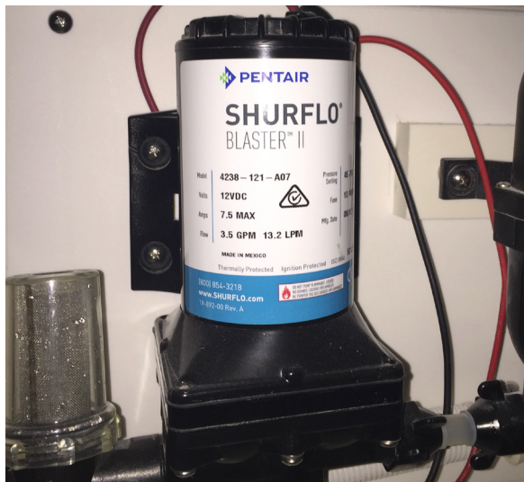
Typical raw water strainer (left) and pump
