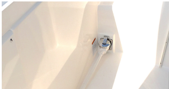
Shore power inlet
