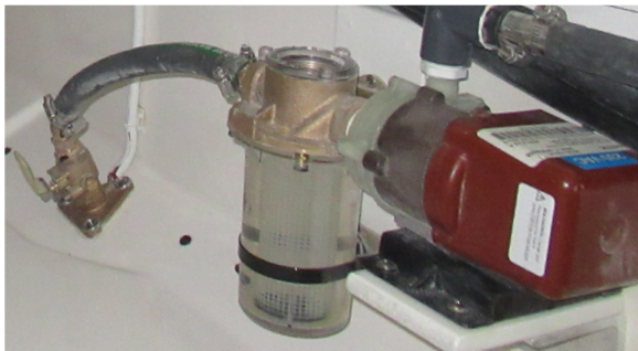
Air conditioning valve, strainer, and pump
