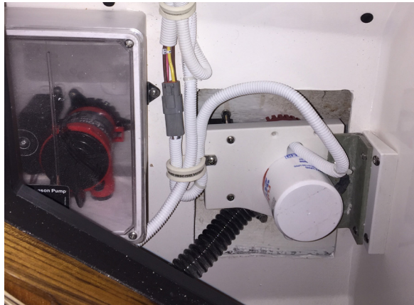
Shower sump box (left) and bilge pump
