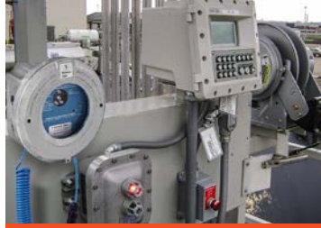
Grounding & Control Systems
