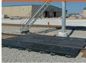
3 RAILCAR TRACK PAN AND SPILL CONTAINMENT
