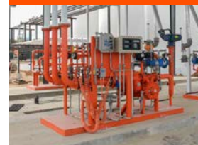
19 BLENDING, METERING AND LOADING SKID
