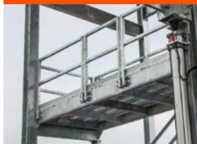
12 METAL HANDRAILS AND CUSTOM PLATFORM
