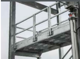
8 METAL HANDRAILS AND CUSTOM PLATFORM
