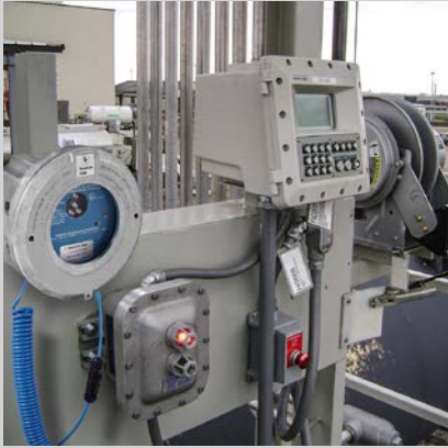
Grounding & control systems
