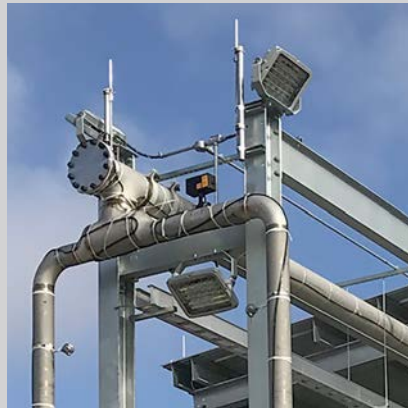
Safety and inspection lighting
