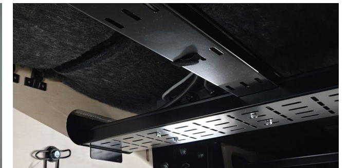
Cable-management within ceiling
