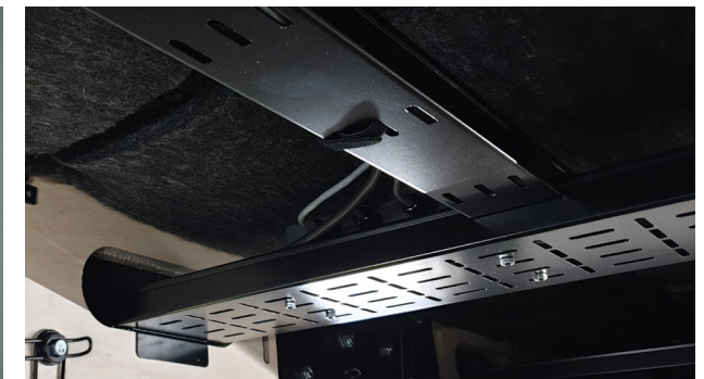
Cable-management within ceiling
