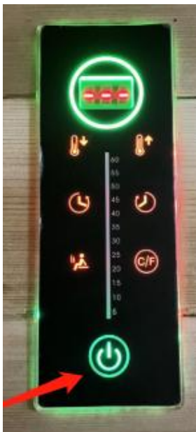
Sauna Control Panel is Illuminated
