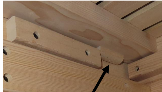
Wood STOP on Underside of BENCH
