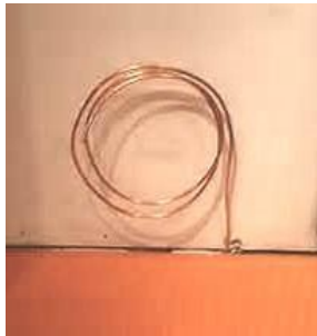
Unapproved Copper water line:
