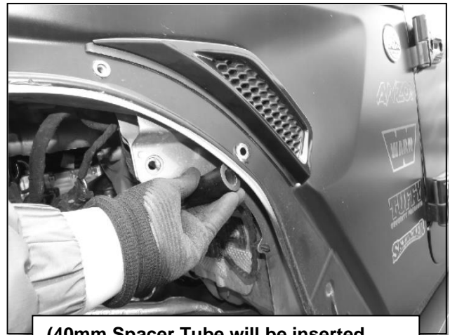
(40mm Spacer Tube will be inserted between upper outer and inner sheet metal when mounting Fender
