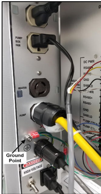
Figure 4-6 Electrical Connections Panel
