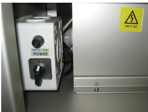
Figure 12 – Power switch location
