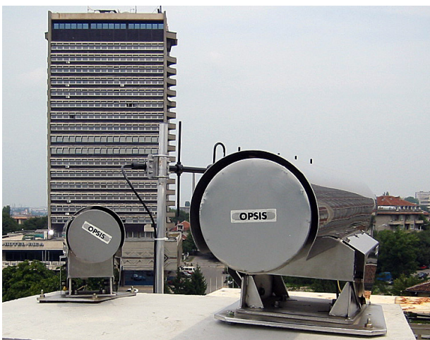
An OPSIS installation at roof-top level
