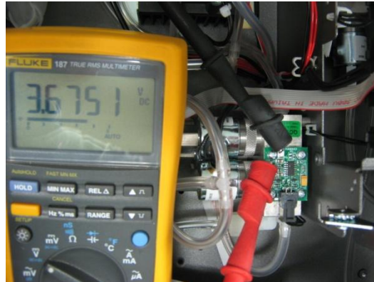
Figure 127 – Typical Test Point Reading of Cell Pressure Sensor
