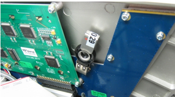
Figure 8 – Installation of USB Memory Stick
