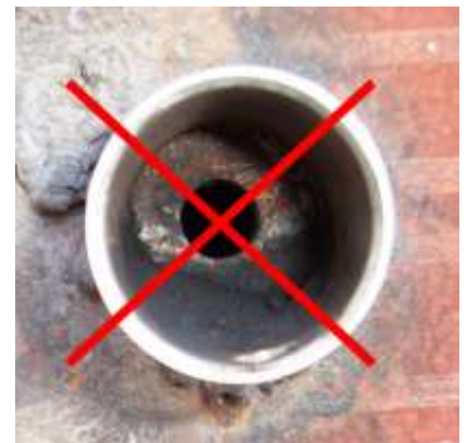
Figure 8 Wrong socket installation
