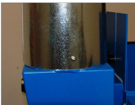
Figure 4. Exhaust Ventilation on Blower Motor's Outlet Flange
