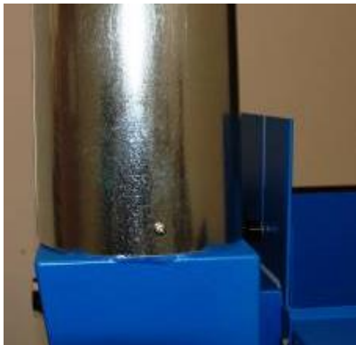
Figure 10. Secure Exhaust Ventilation Stack
