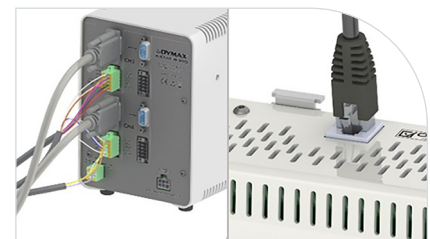
From this wiring
