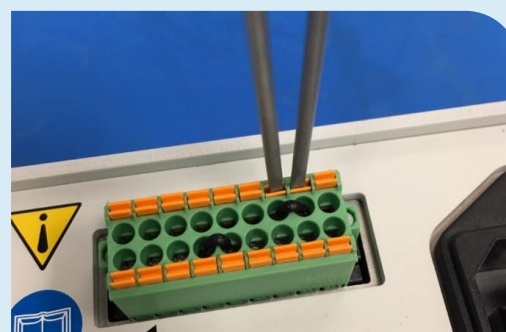
Figure 11. Remove Jumper from Terminal Block
