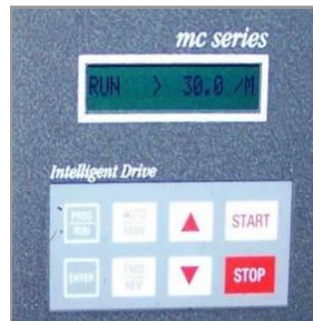
Figure 12. Conveyor Speed Controller
