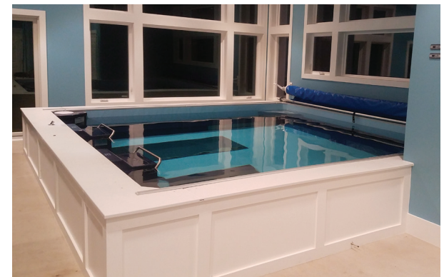
Partially In-Ground Indoor Installation
