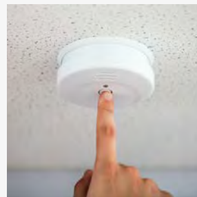
Smoke Alarm Compliance $129 Annually
