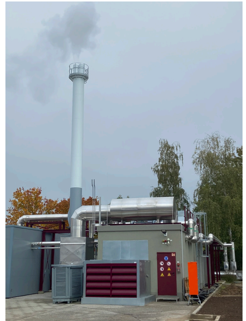
Geothermal power plant
