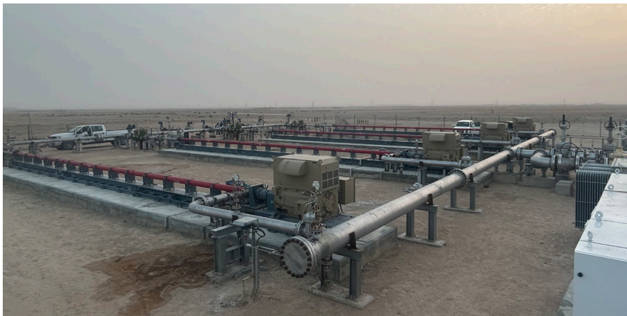
Four Hercules SH13500 HPS run in parallel.
