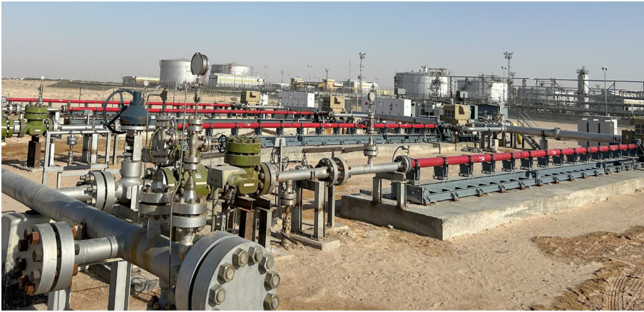
Hercules SH13500 HPS with minimal infrastructure footprint.
