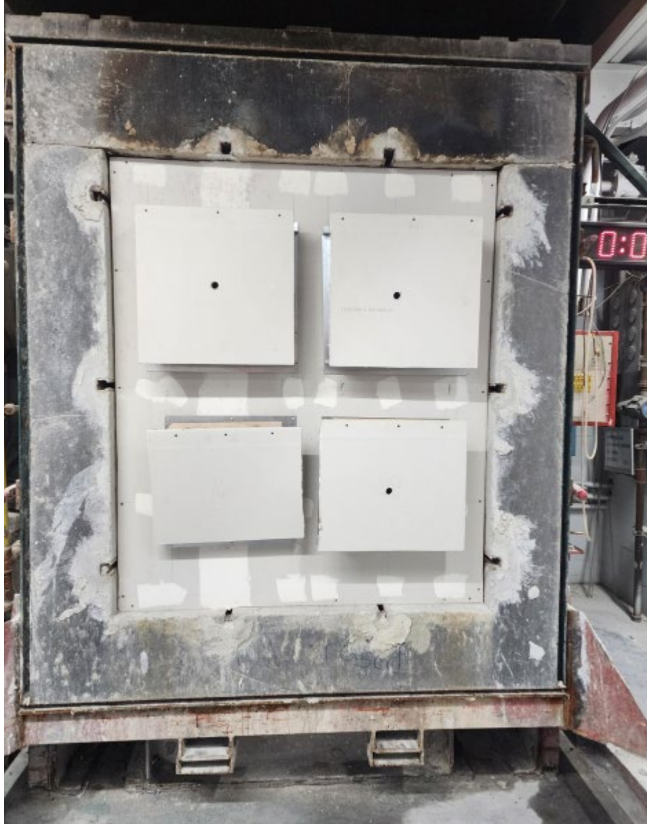
DAMPERS COVERED PRIOR TO THE START OF THE FIRE EXPOSURE
