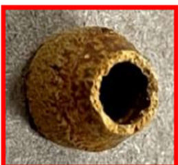
Leaking Ferrule: pitted and chipped surfaces (cleaned with harsh chemicals)
