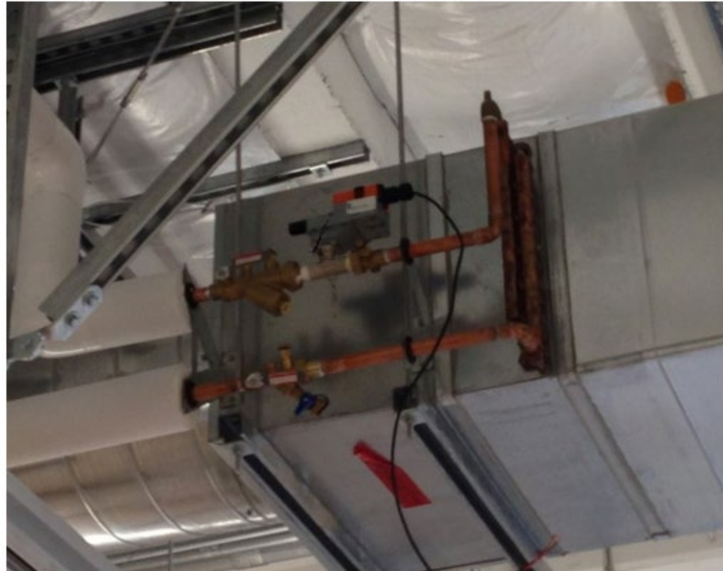
VAV REHEAT COILS
