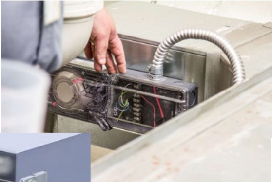
DUCT SMOKE DETECTORS
