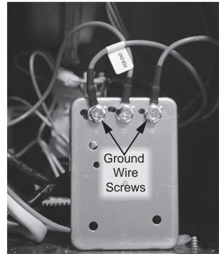
Figure 54 - Location of ground wires
