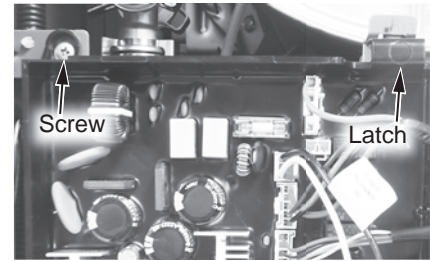
Figure 63 - Control board location
